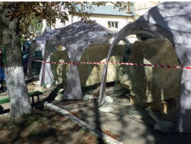
Delivery of the rocks for the new stonemasonry workshop at the courtyard grounds of the Ivan Trush College, 2017
